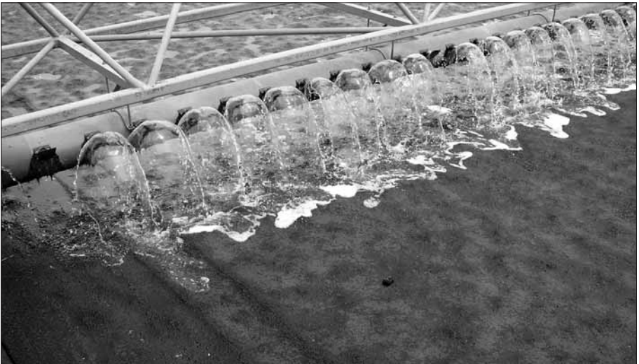
Figure 19.3 Rectangular Biofilters Covered with High-density Polyethylene Netting to Control Fly Nuisance
